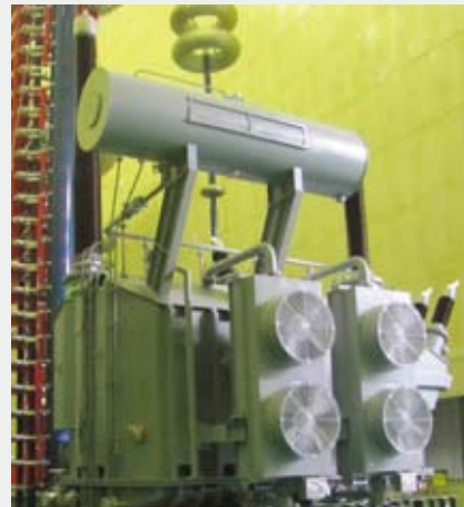
衡变——南网桂林变电站 ODFPS-250MVA/500KV Hengyang transformer-Guilin transformer substation of China Southern Power Grid ODFPS-250MVA/500KV
