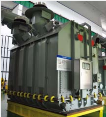
沈变——糯扎渡水电站 DSP-241MVA/500KV Shenyang transformer-Nuozhadu hydropower station DSP-241MVA/500KV
